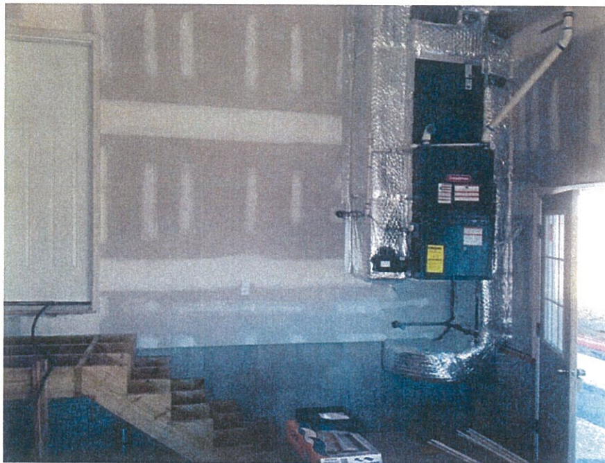
4 Bluebeard Drive, Lowest Utility Duct work, 11/25/13
